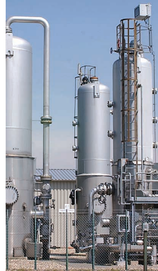
Gas storage facility Kalle Germany, © RWE
