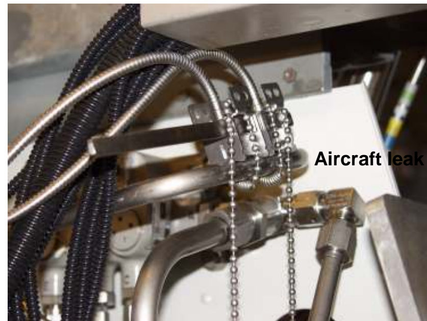
High pressure, small pipes
