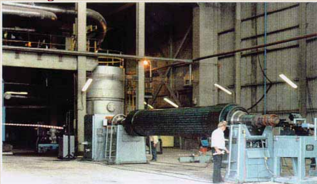
Generator rotor - service work at site included re-grinding of collector rings with machining attachment and low-speed trim balance.
